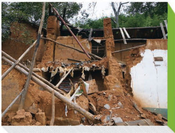
Figure 1: Local traditional rammed earth building destroyed by earthquake
